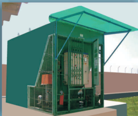
A standard Packaged KDBR system installed in an educational institute in India.
